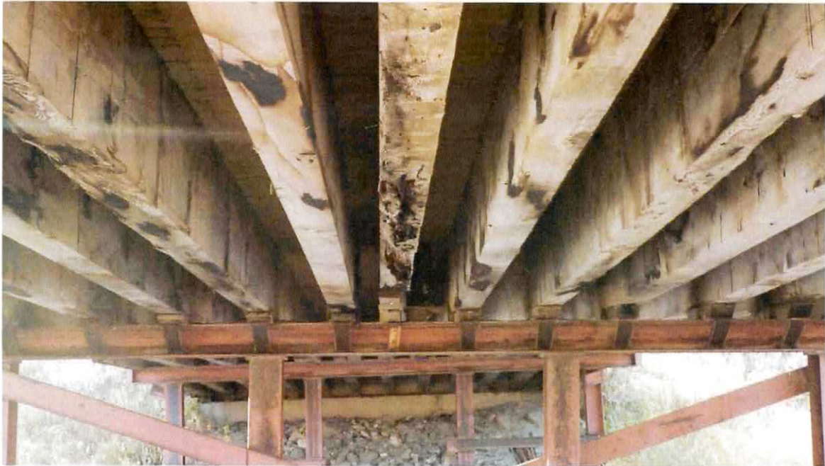
G7 span 2, NOTE: Rot along underside of G7
