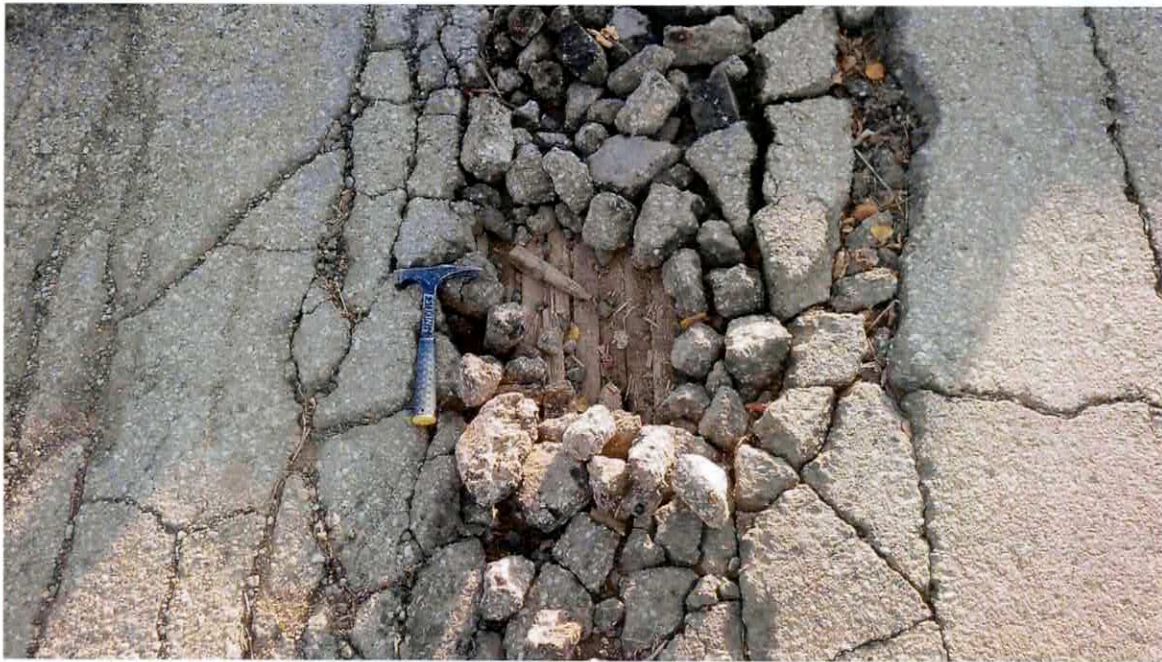
Looking over SU2. NOTE: Missing asphalt with exposed deck boards (2)
