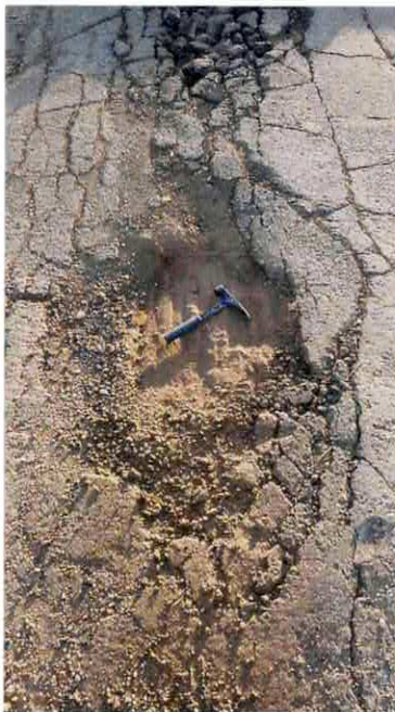
Looking over SU2. NOTE: Missing asphalt with exposed deck boards (1)
