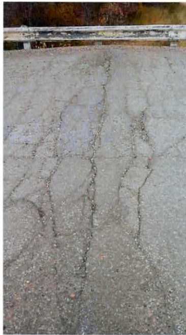
Looking East over SU4. NOTE: Alligator cracking caused by differential movements and pier heaving
