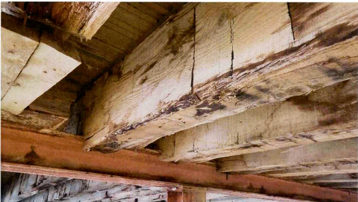
G6 span 1, NOTE: Splitting at end notch
