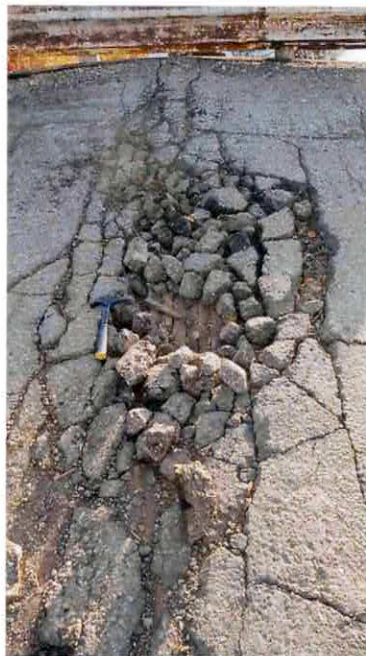
Looking over SU2. NOTE: Missing asphalt with exposed deck boards (3)
