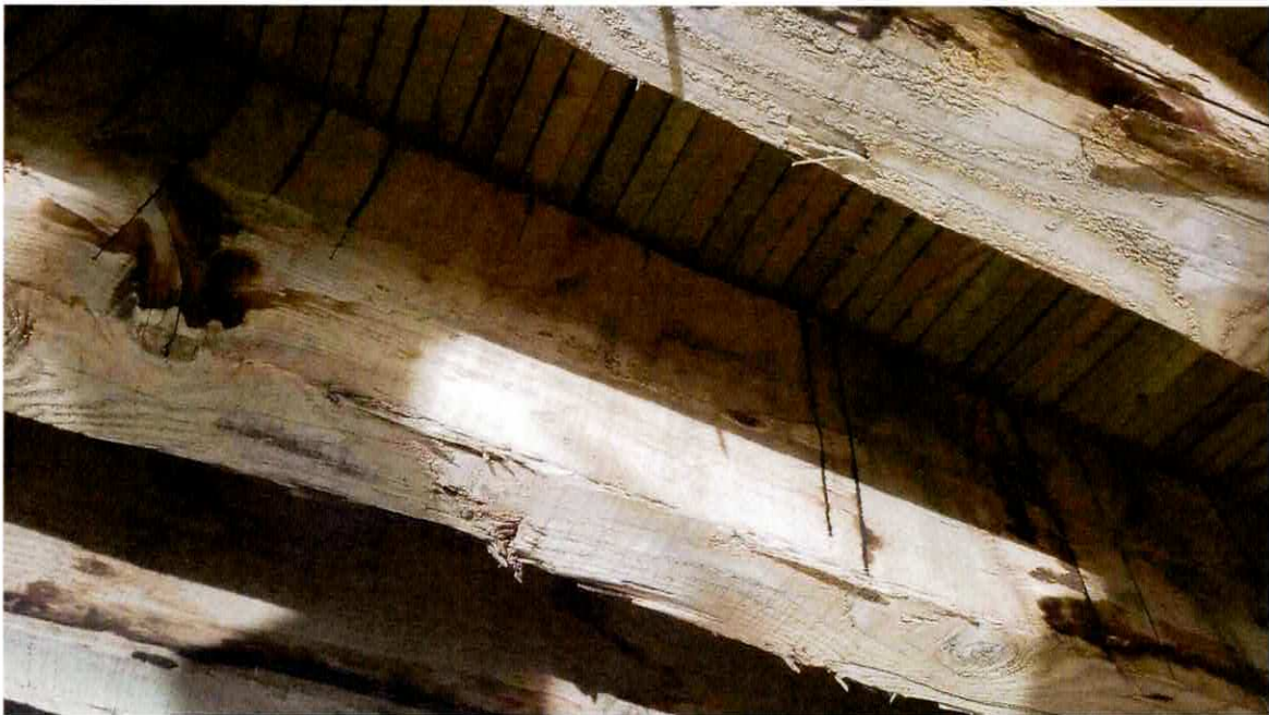
Span 2 minor girder defects
