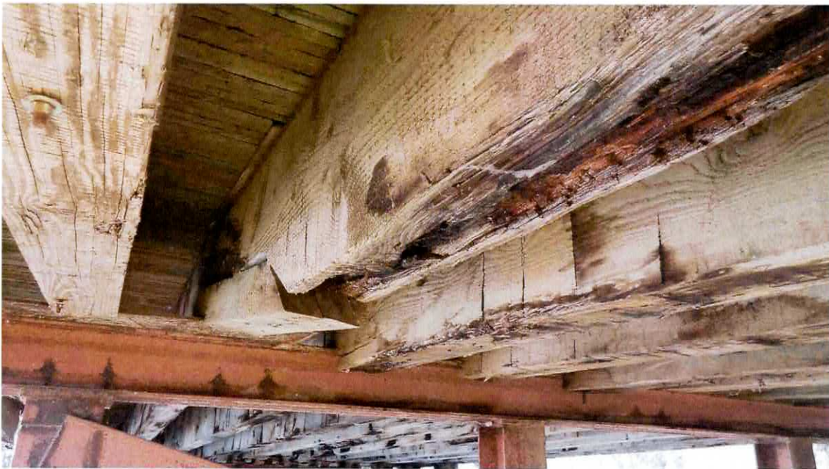
G5, span 1. NOTE: Rotten along under side and splintered at SU2.
