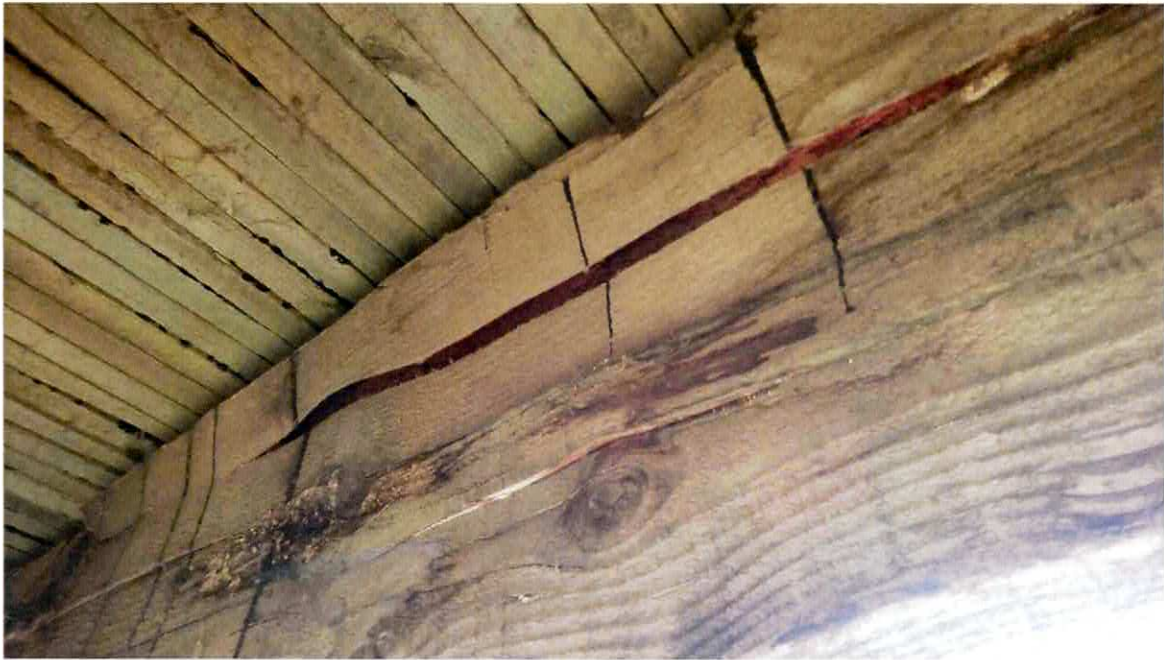
G13, span 1. NOTE: Severe rot
