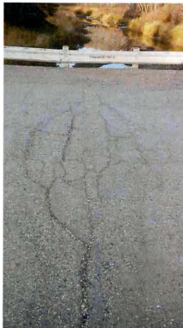
Looking East over SU3. NOTE: Alligator cracking caused by differential movements and pier heaving
