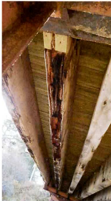
G2, span 2. NOTE: Rotten along underside
