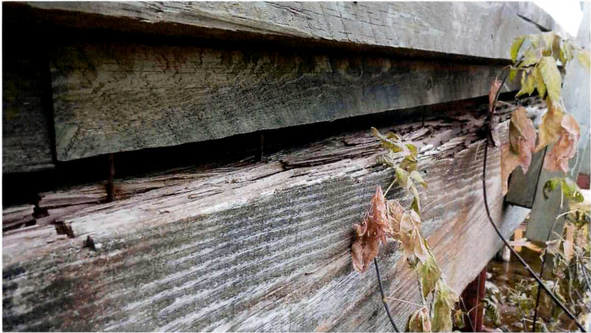
G1, span 4. NOTE: Rotten, full depth (2)
