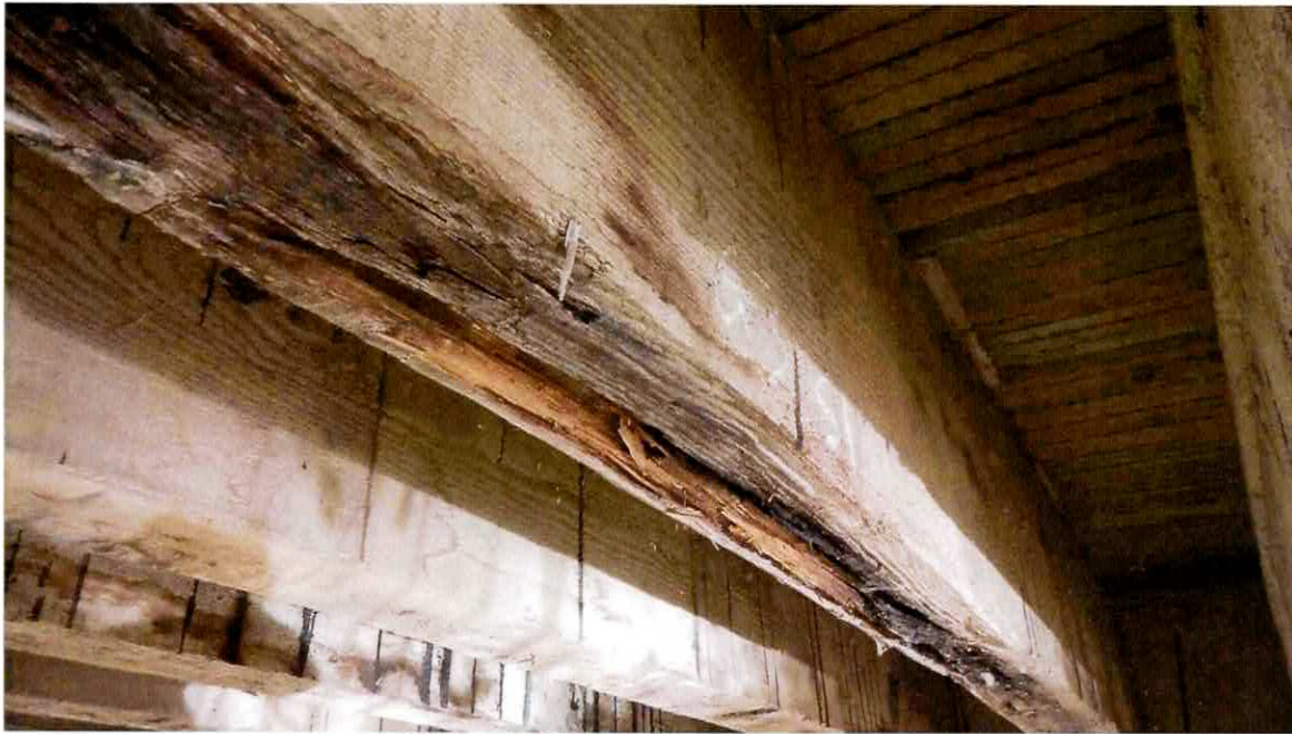
G5, span 1. NOTE: Severe rot along underside
