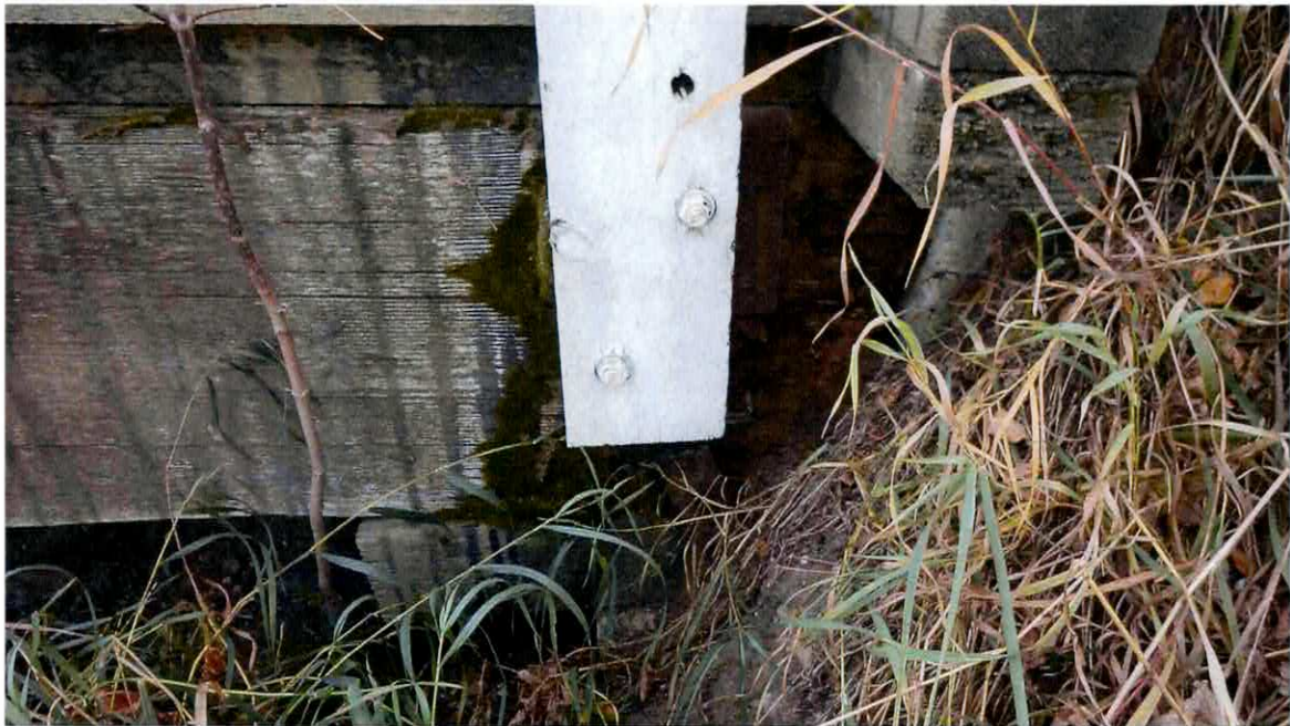
G13, span 4. NOTE: Severe rot over abutment
