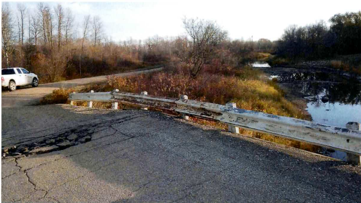
Showing heaving at SU2, East side
