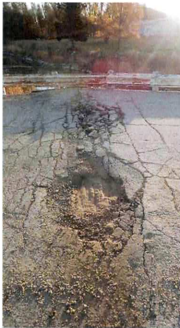
Looking East over SU2. NOTE: Severe asphalt damage and exposed deck boards
