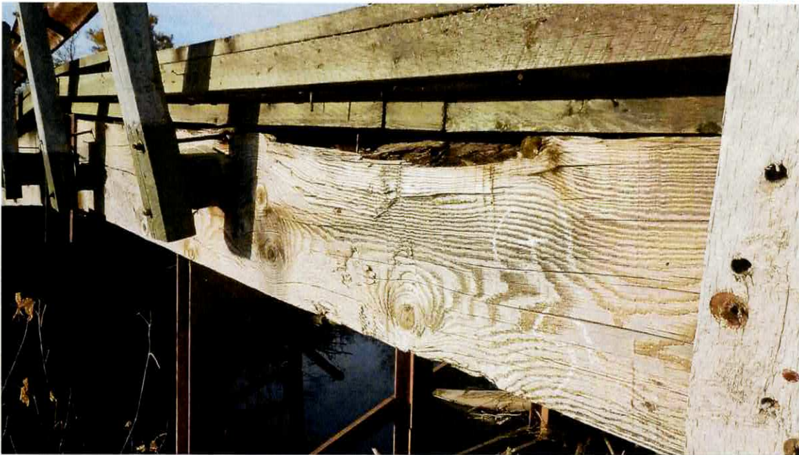
G1, span 1. NOTE: Severe rot throughout (1)
