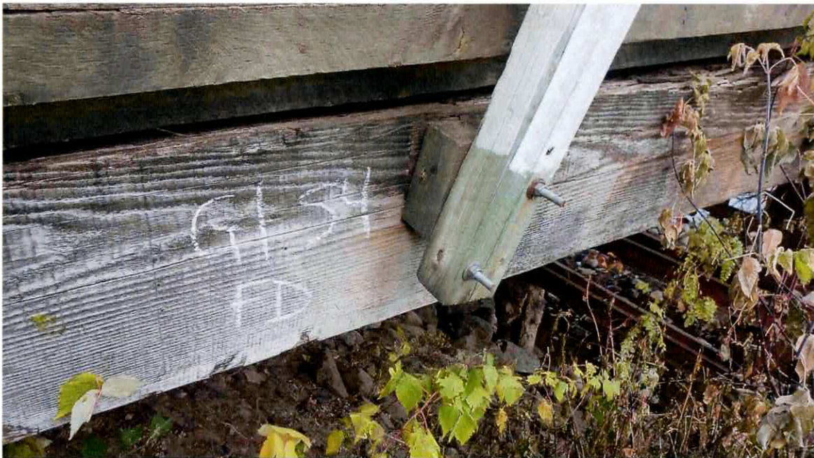
G1, span 4. NOTE: Rotten, full depth (1)
